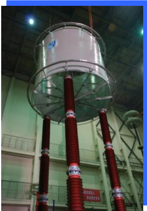
500kV shunt reactor supporting composite post with porcelain core
